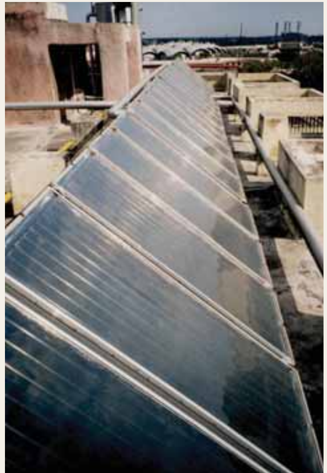
Solar collectors for heat water supply at the headquarters of the All India Womens Conference in New Delhi. Photo: Kirsten Ulsrud.
